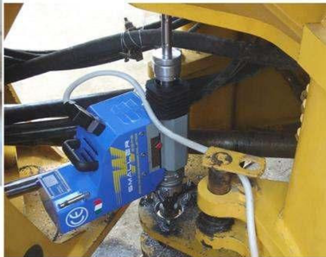
Reconditioning and realignment of the central articulation of a wheel loader. The work is carried out directly on site without disassembling the hydraulic tubes, thus avoiding waste of oil and respecting the environment.
